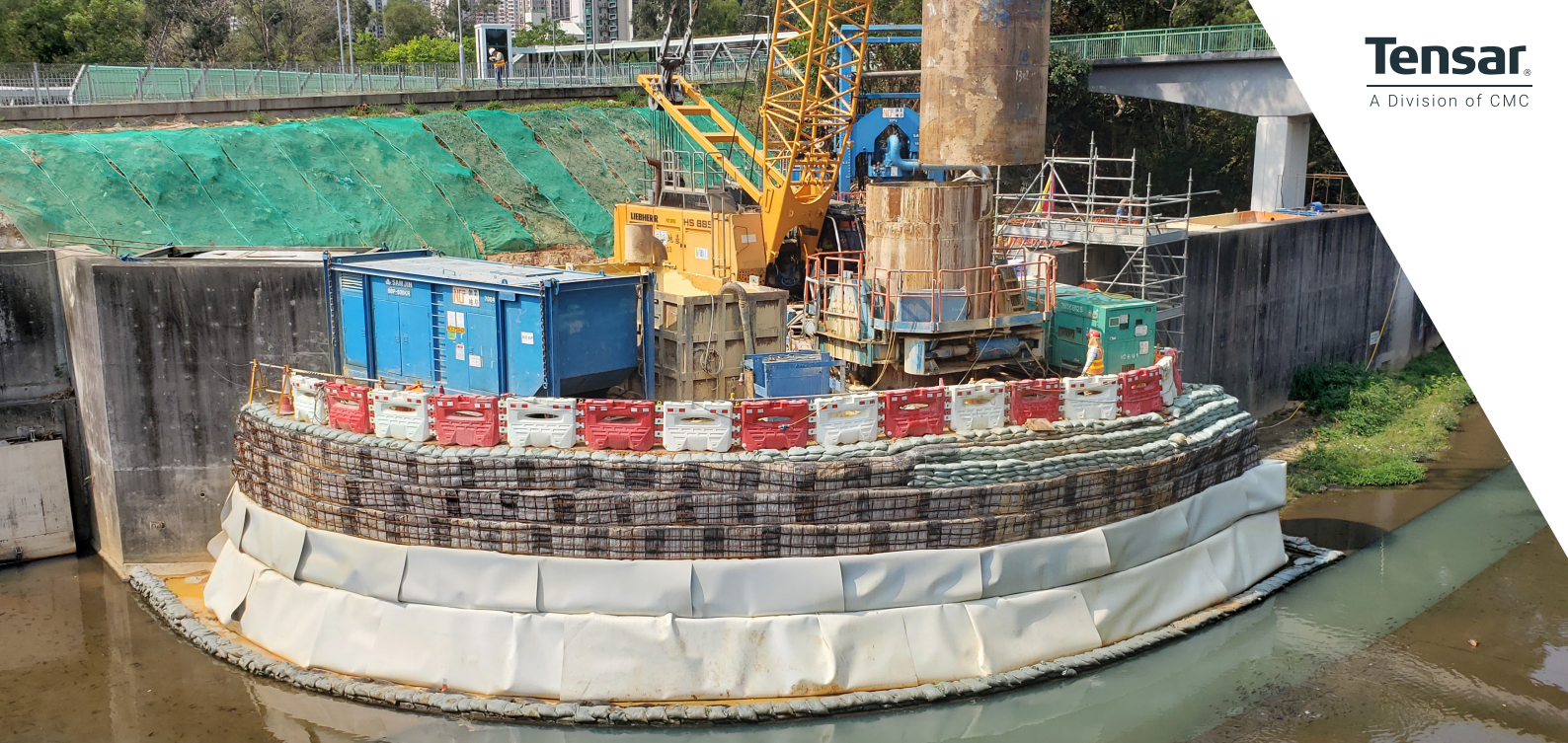
Completed reinforced soil structure (RSS) as a working platform at service stage
